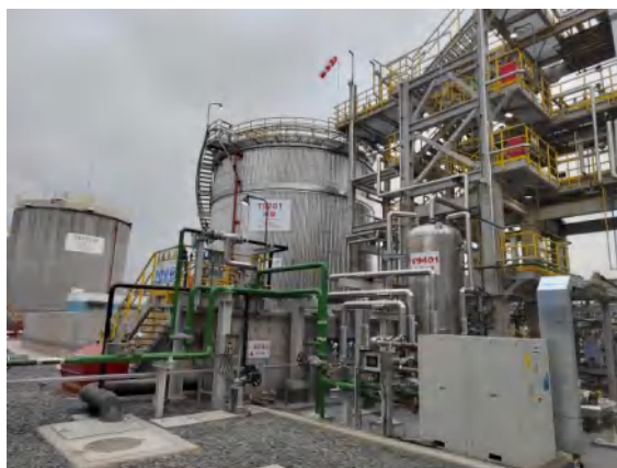
新建丙醛储罐和冷冻水缓冲罐
